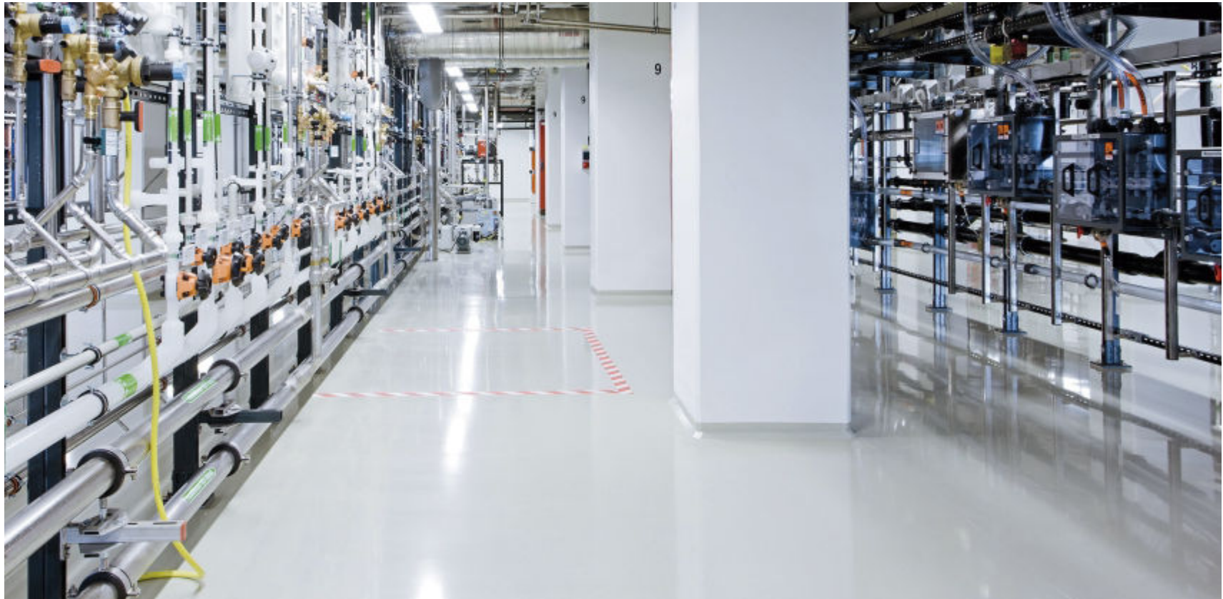
Sika flooring for Fraunhofer IPA*, Germany
